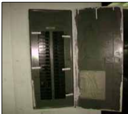
SUB PANEL #1 AREA DE CAFETERIA
